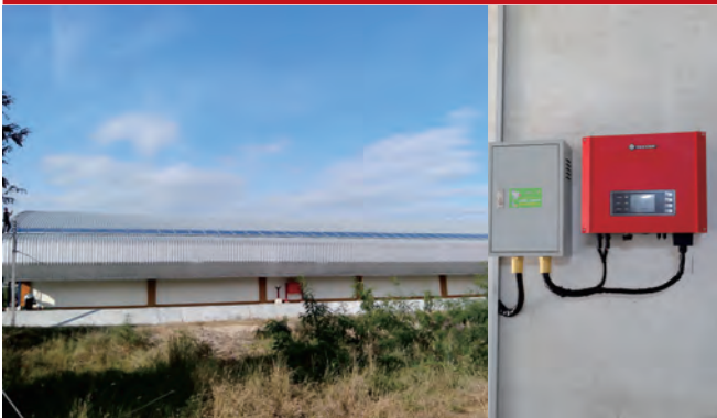
10kW, 2pcs 5kW, Thailand
